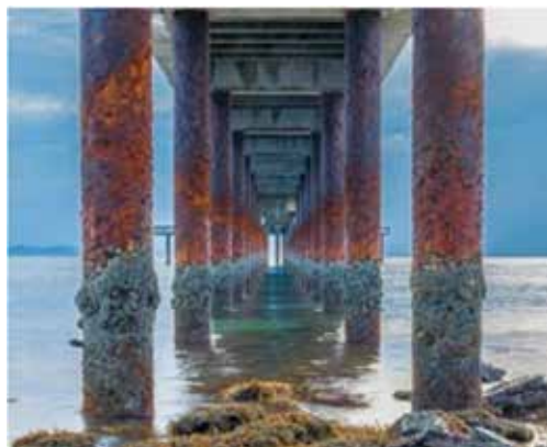
The very attractive rusting pylons holding up our magnificent pier.
